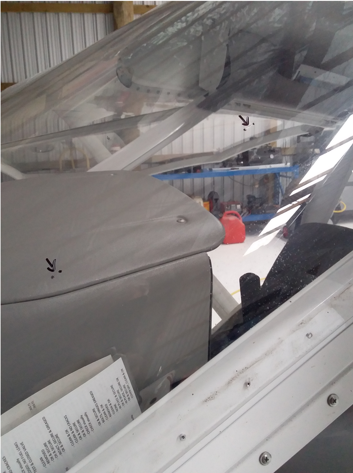
Photo 1: Windscreen LH side – Upper and lower cracks found in an A-32 windscreen. (The location of the two small cracks are between the dots and marked with black arrows).
