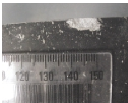
Watch for signs of corrosion, such as those pictured above, and seek the advice of a LAME if in any doubt.
