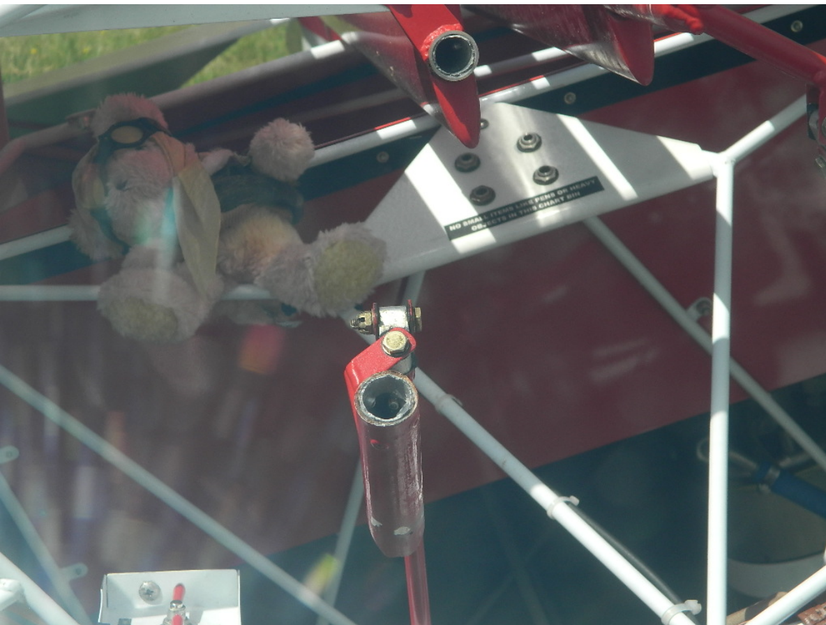
Photo 2 – A closer view of the failed starboard flaperon control rod.
