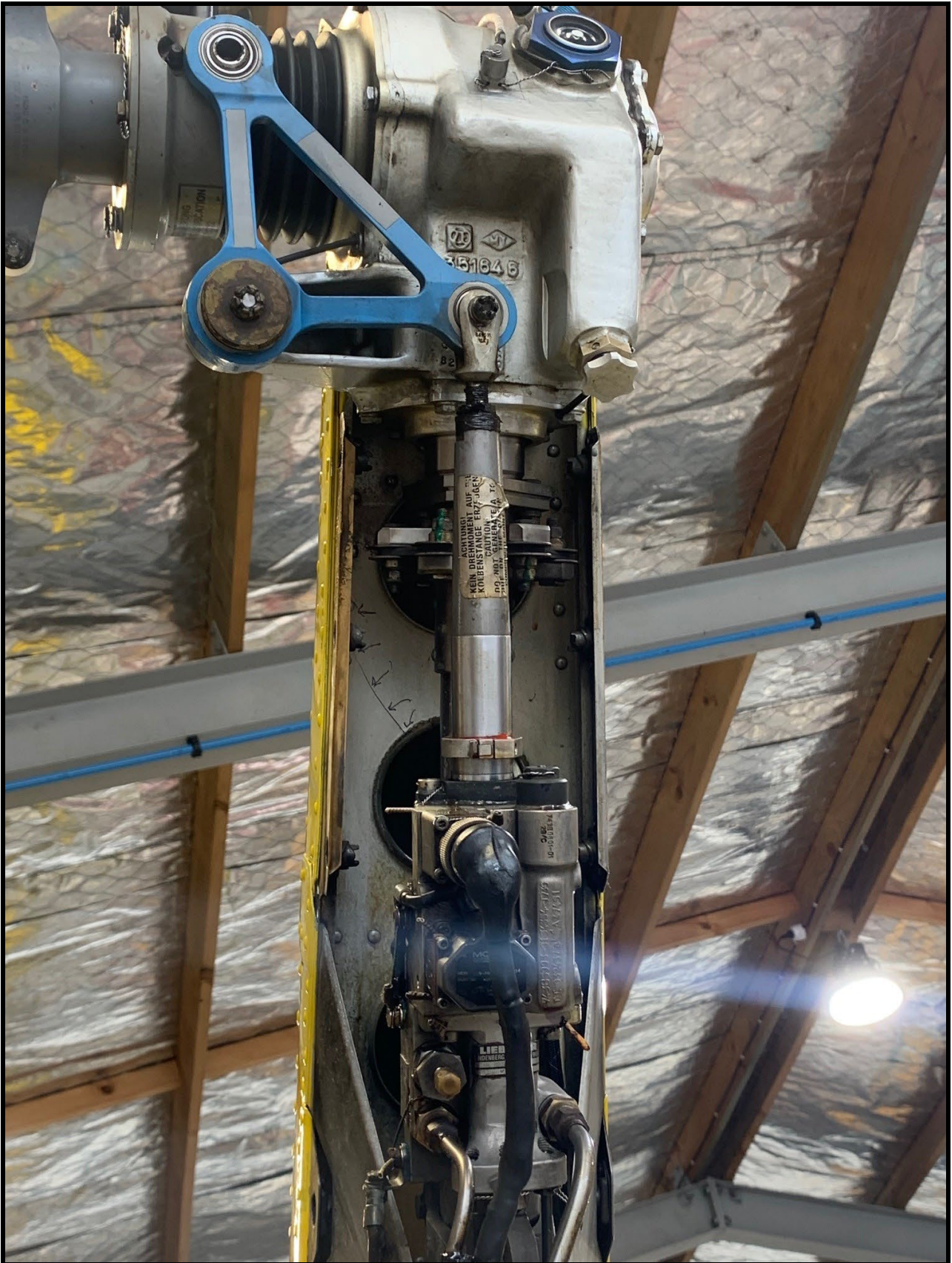
Photo 1: Location of crack found in vertical fin spar.
